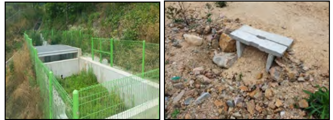
Figure 1: overgrown vegetation and soil inflow
